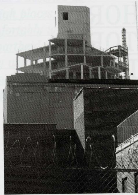
Luxury condo construction at 525 Clinton Ave. in Brooklyn, NY, March 2007. Photo: Punam Khosla.
